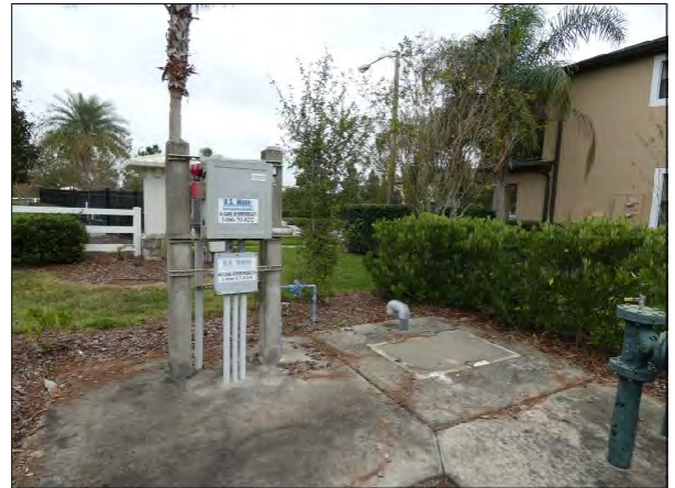
Meadow Pointe North Lift Station
