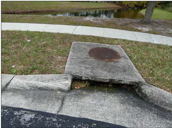
Stormwater Drainage Curb Inlet
