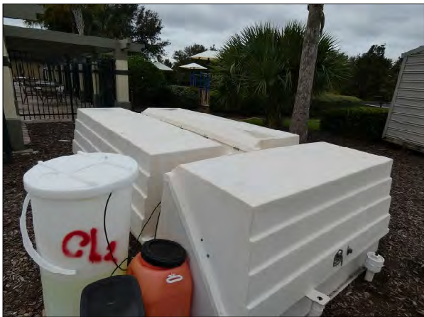
Pool Equipment Housing Boxes
