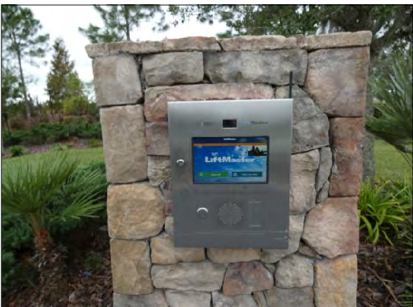
Typical Gate Key Pad
