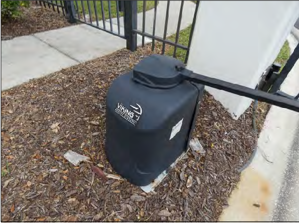
Typical Gate Operator
