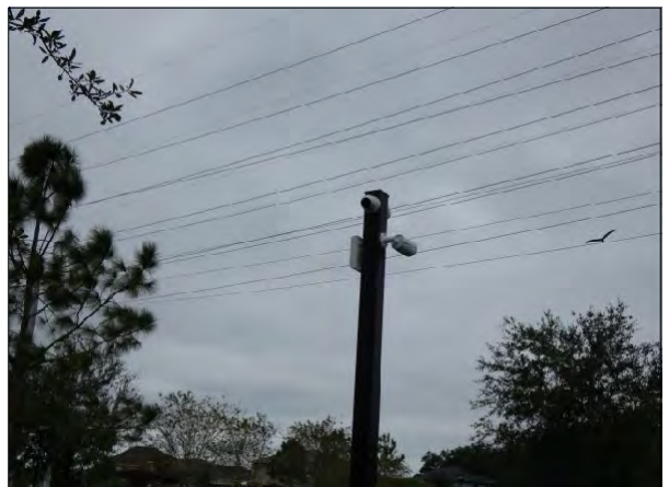
Typical Gate Camera System
